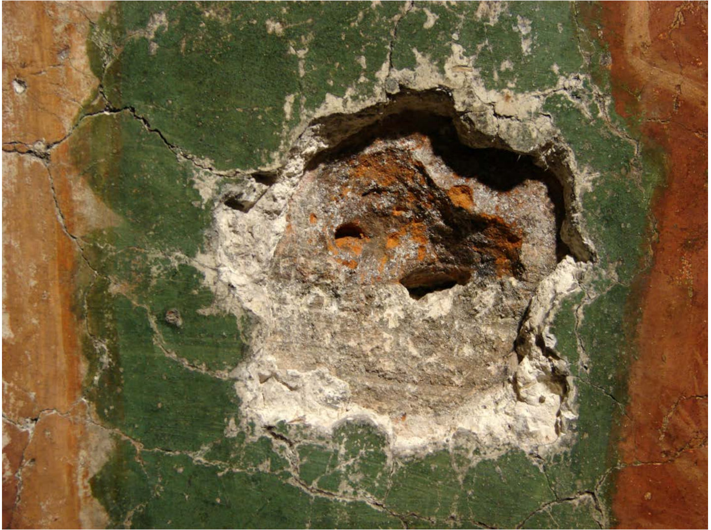
Missing part of painted plaster, Arbore Church (Romania), 1502; Photo: 2006, UAD (Theo-Sandu Mureşan)
