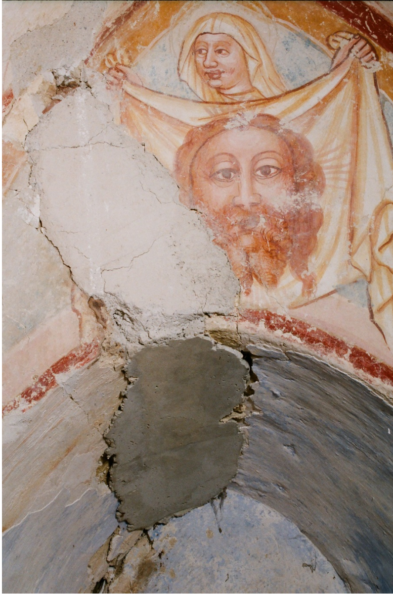
Incorrect plaster application, Chapel of St. John the Baptist, Ivanić Miljanski (Croatia), ca. 1450; Photo: 2002, HRZ (Ivan Srča)
