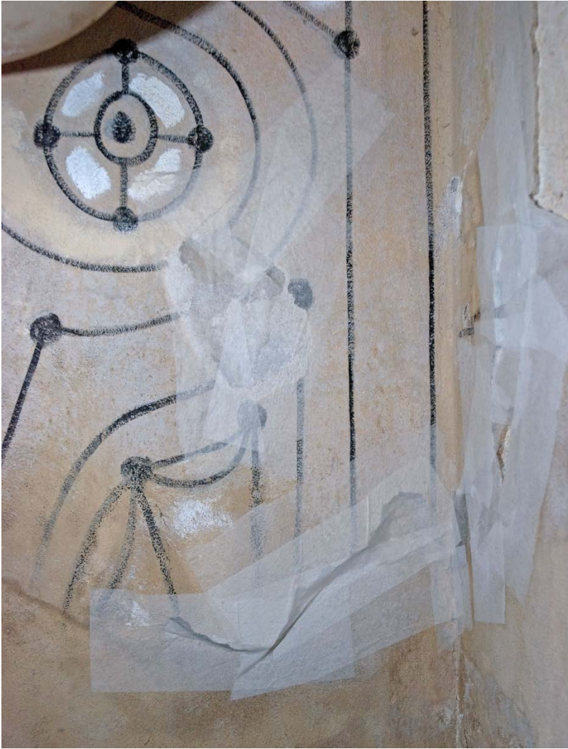
Facing applied to temporarily prevent scaling and delaminated areas from falling, chapel Saint Pierre, Villefranche sur mer (France), painted by Jean Cocteau, 1956/7; Photo: 2008, CICRP (Odile Guillon)
