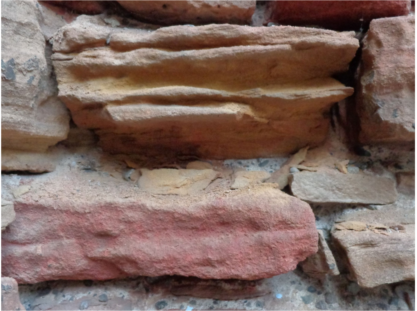
Loss of material caused by wind erosion, Dominikanerkirche, Colmar (France), 1289–1346; Photo: 2015, RPS (Dörthe Jakobs)
