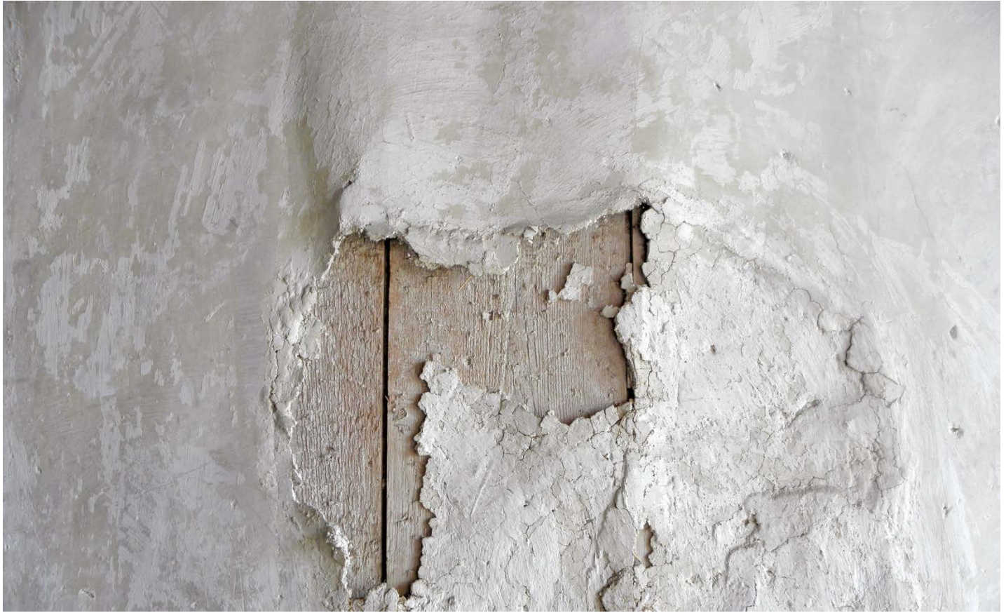
Fragmentary whitewash on damaged plaster layer, Çeyrekçiller House, Safranbolu (Turkey), 19th century; Photo: 2012, KBU (Aysun Özköse)
