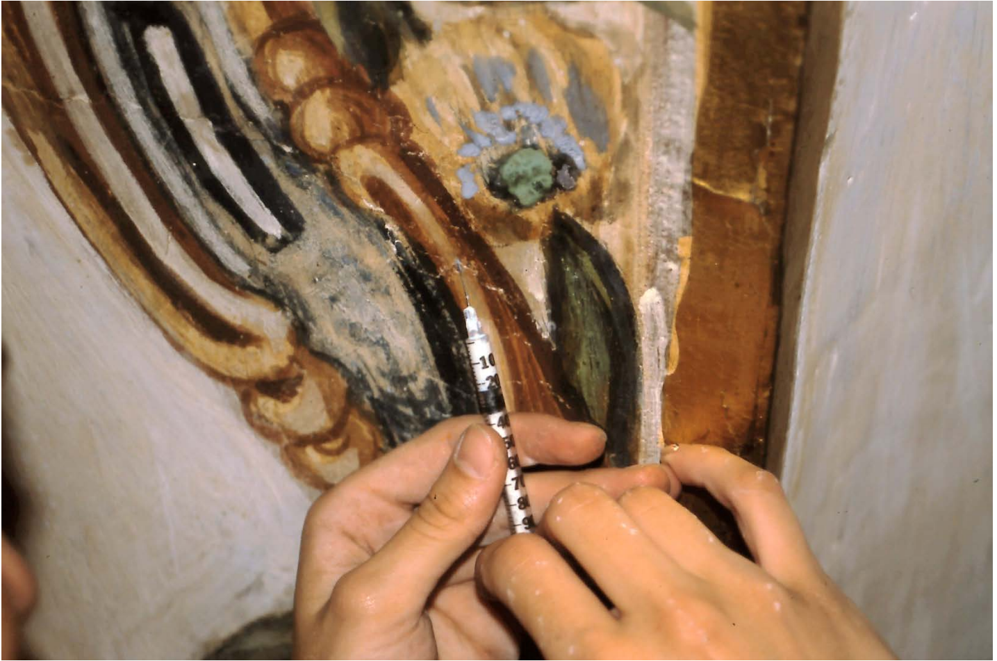
Injection of an adhesive into a wall painting, Church of San Roque, Oliva (Spain), 20th century; Photo: 2009, UPV
