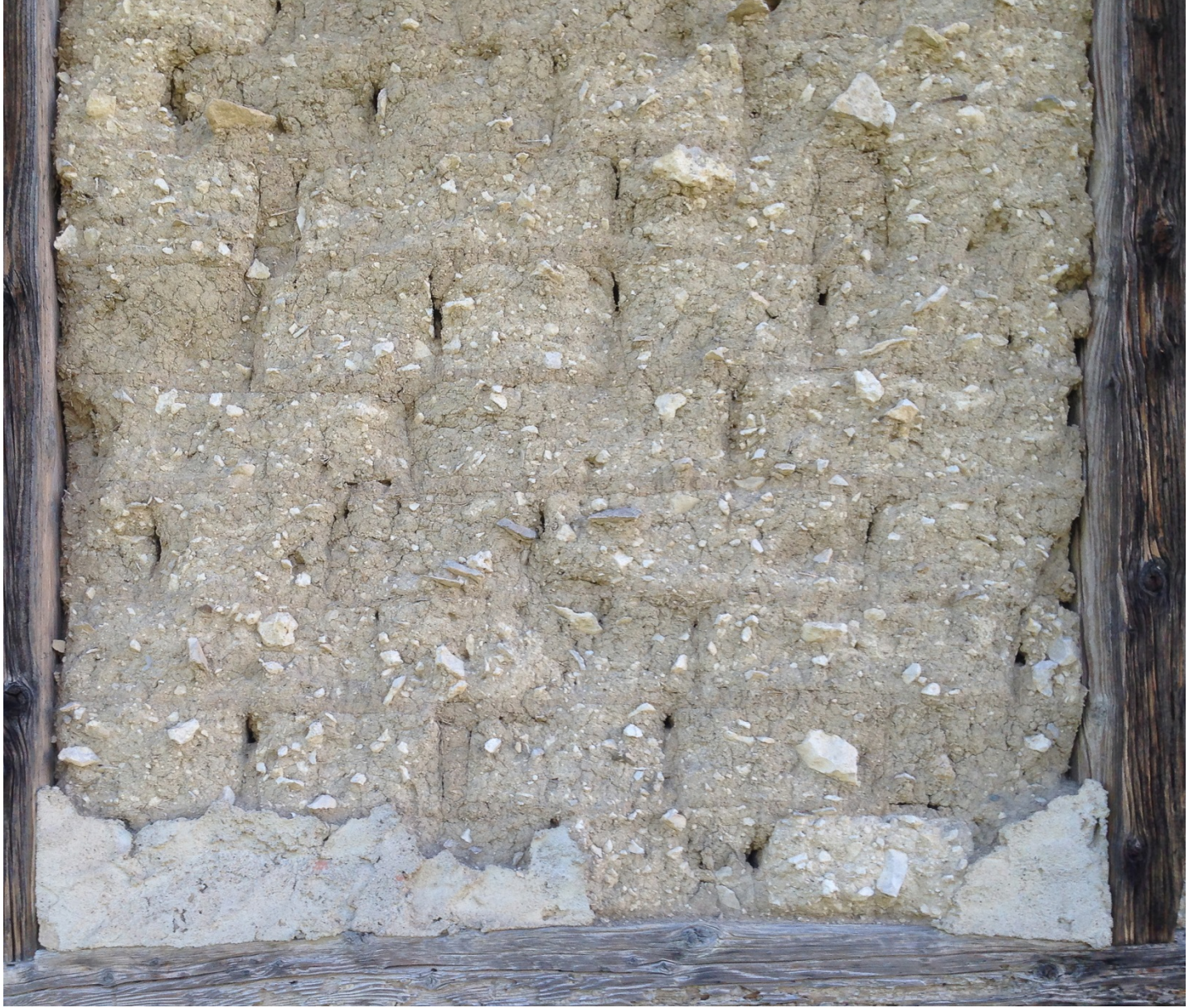
Half-timber construction with adobe, Yourk village of Safranbolu ( Turkey), 19th century; Photo: 2014, KBU (Eray Şahbaz)
