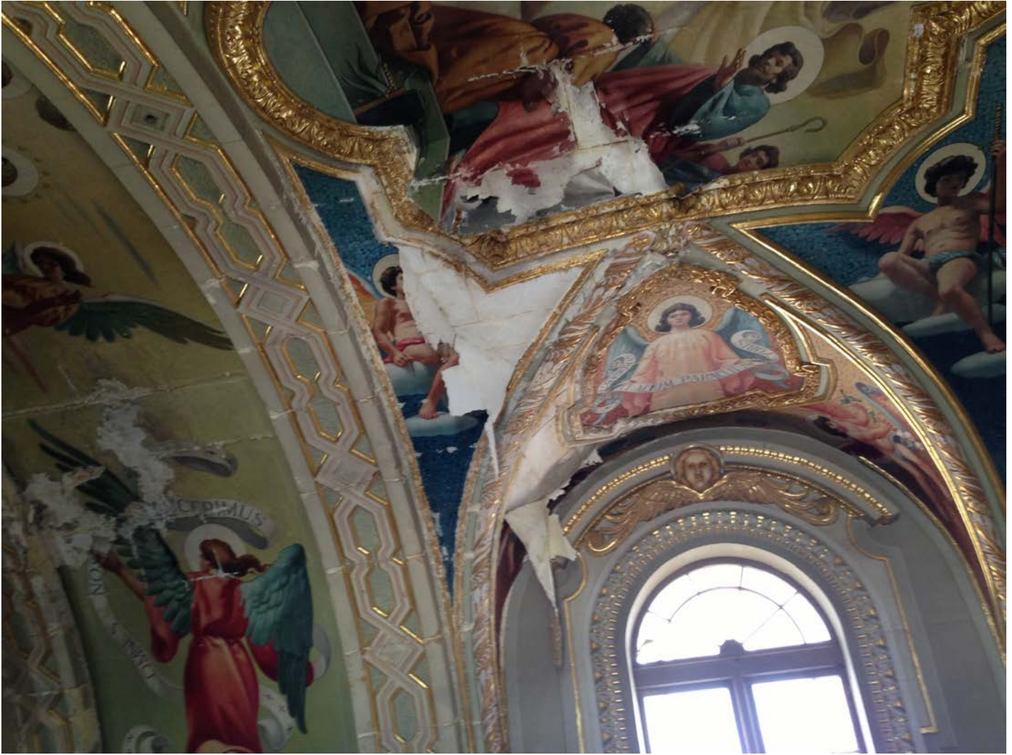
A detached marouflage painting due to the infiltration of water from the roof. Chapel of the Sacred Heart of Jesus, Nadur, Gozo (Malta), 1950s; Photo: 2013, UM (JoAnn Cassar)
