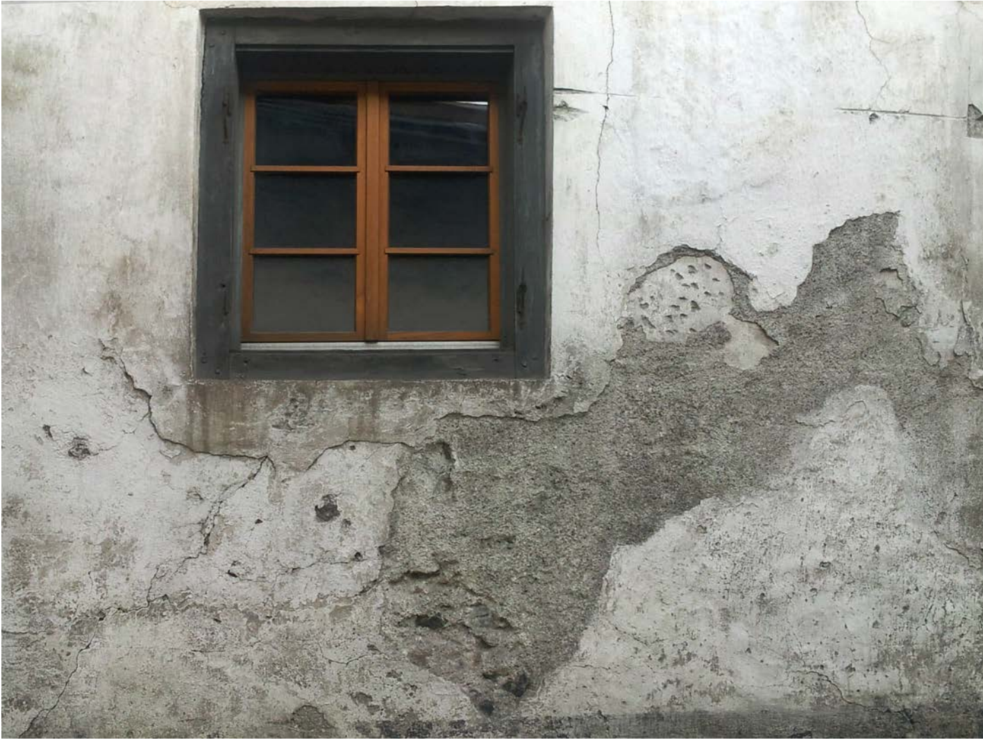
Plaster layers with final render above, historic building, Santa Maria Val Müstair (Switzerland); Photo: 2015, HAWK (Angela Weyer)
