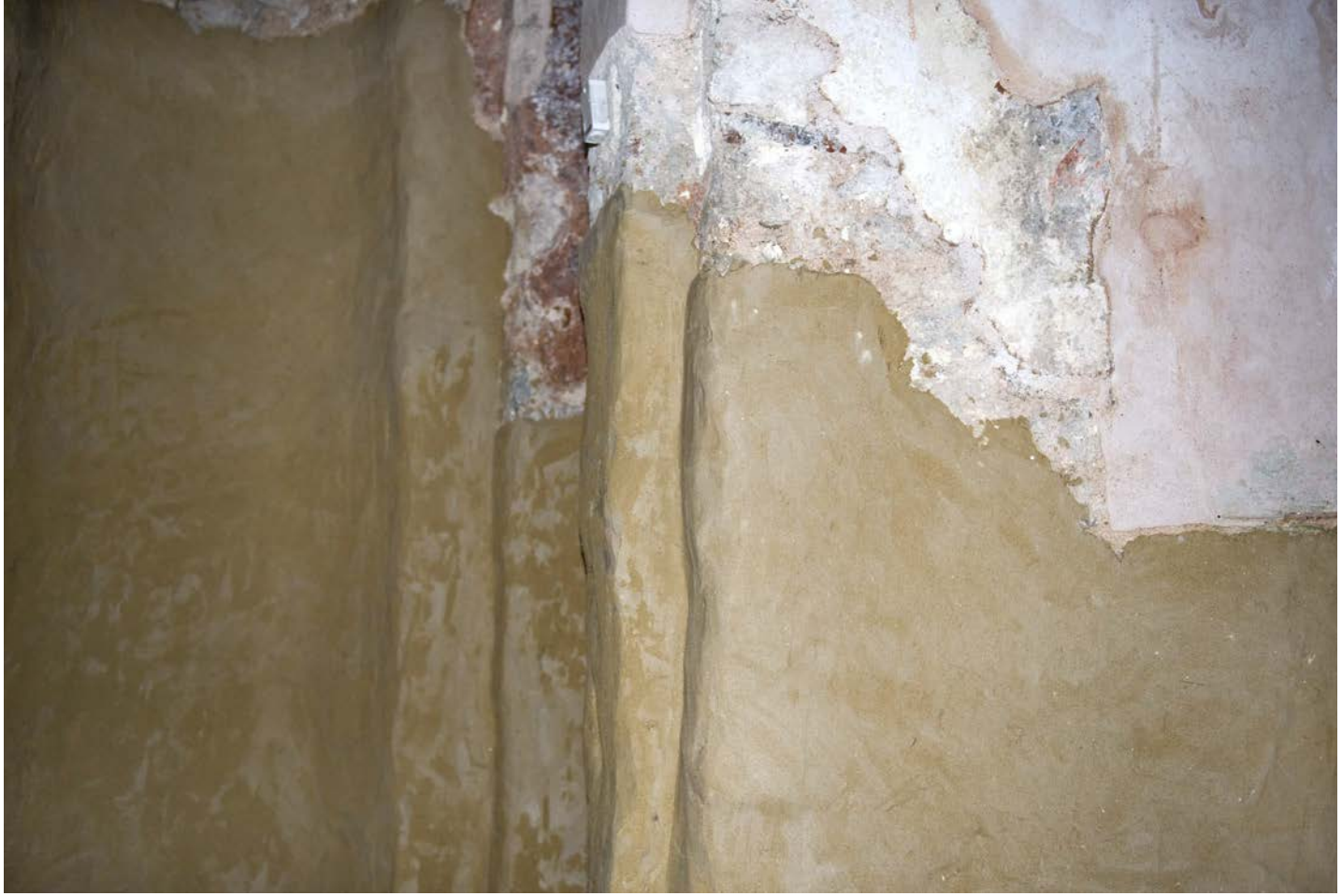
Sacrificial render applied to a wall within the church of St. Michael, Ston (Croatia), 11th century; Photo: 2011, HRZ (Veronika Šulić)
