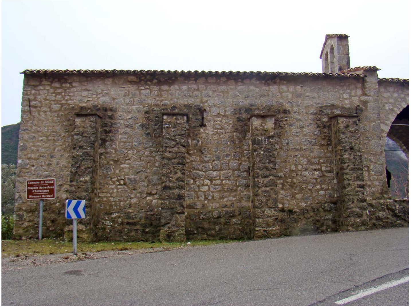
Areas of moisture infiltration are evident as darkened areas, Chapel of Notre-Dame-d'Entrevignes, Sigale (France), 15th century; Photo: 2014, CICRP (Jean-Marc Vallet)
