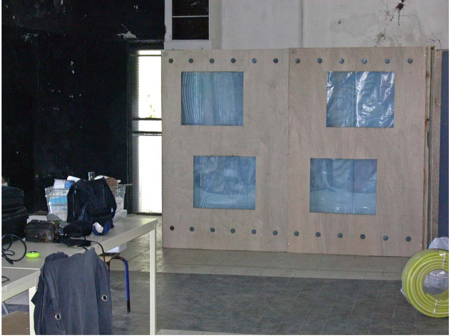
Temporary protection, wall painting by Le Corbusier during restoration of Villa E-1027, Roquebrune-Cap Martin (France), 20th century; Photo: 2007, CICRP (Odile Guillon)
