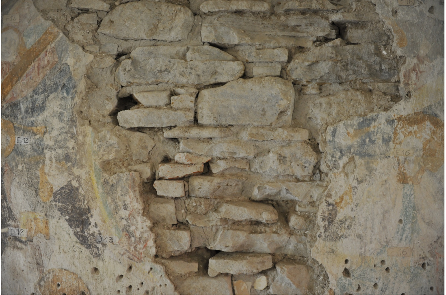
Loss of plaster shows masonry support (detail), Fortified Church in Apold (Romania), 13th century; Photo: 2014, UAD (Adrian Rauca)
