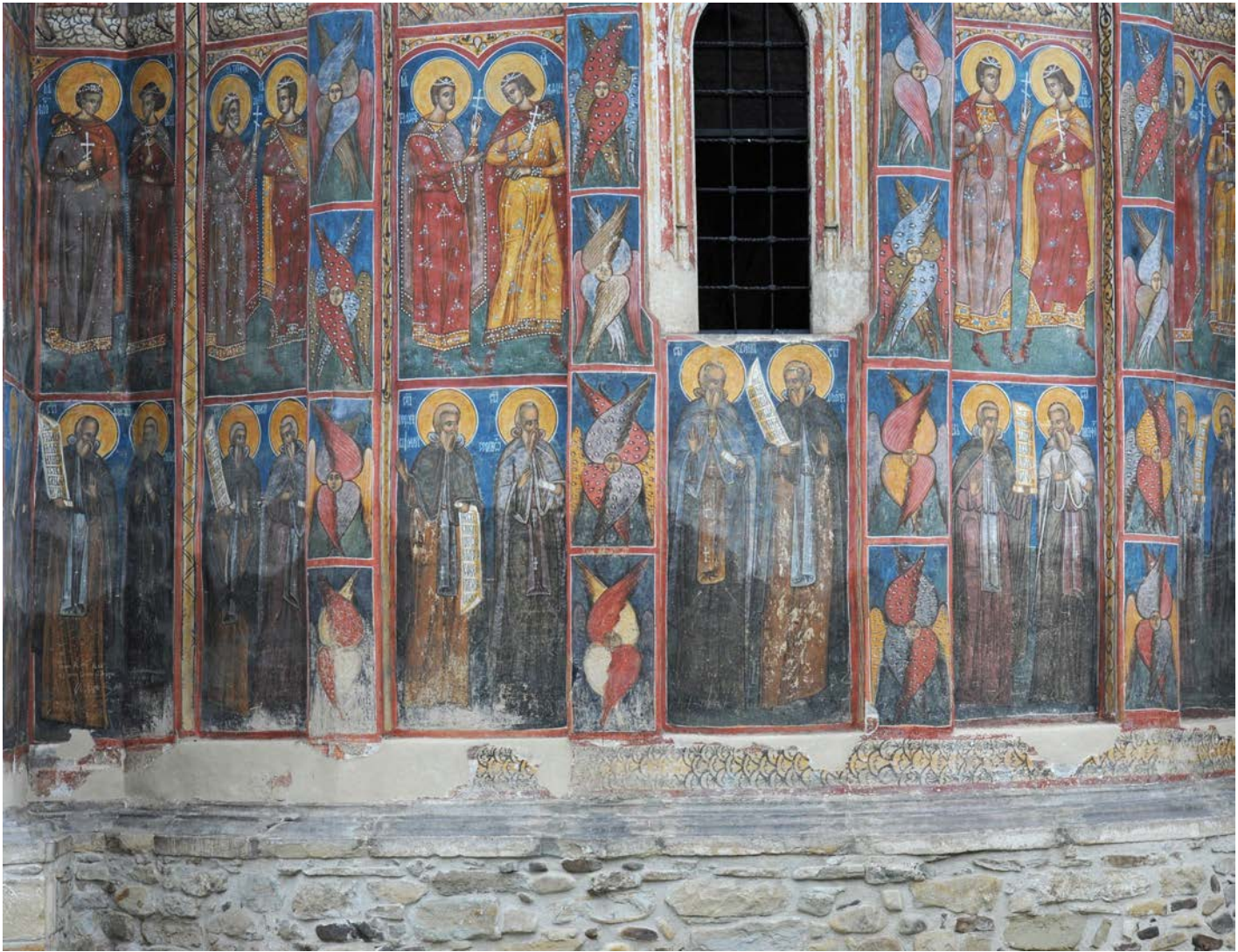
Rising damp visible as colour saturation, Moldovița Monastery (Romania), 1532; Photo: 2003, UAD ( Theo-Sandu Mureșan)
