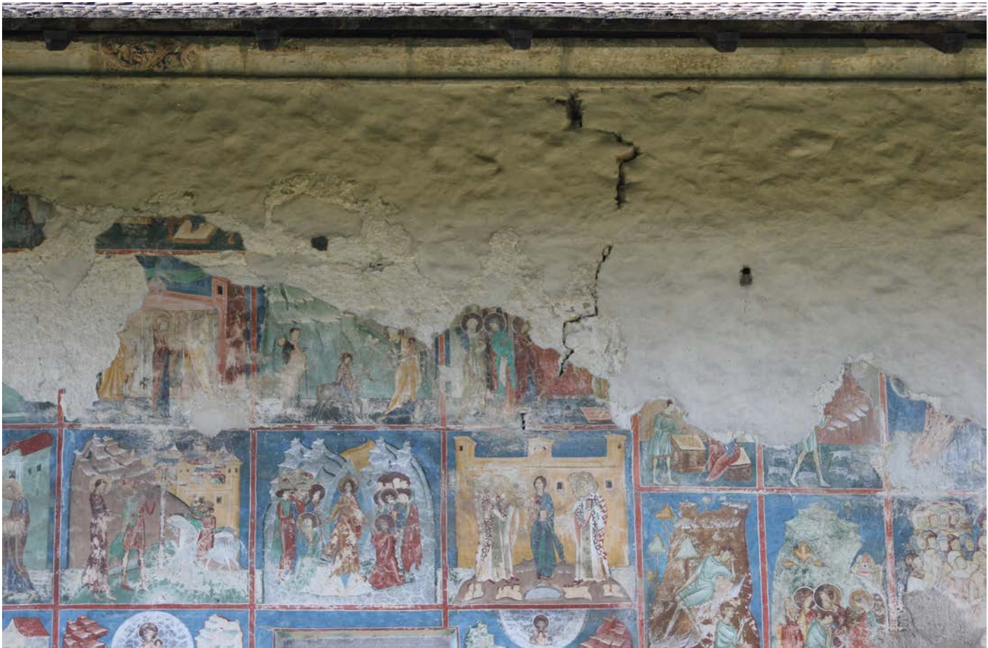
Crack caused by structural movement of a building, Arbore Church (Romania), 1502; Photo: 2012, UAD (Adrian Rauca)
