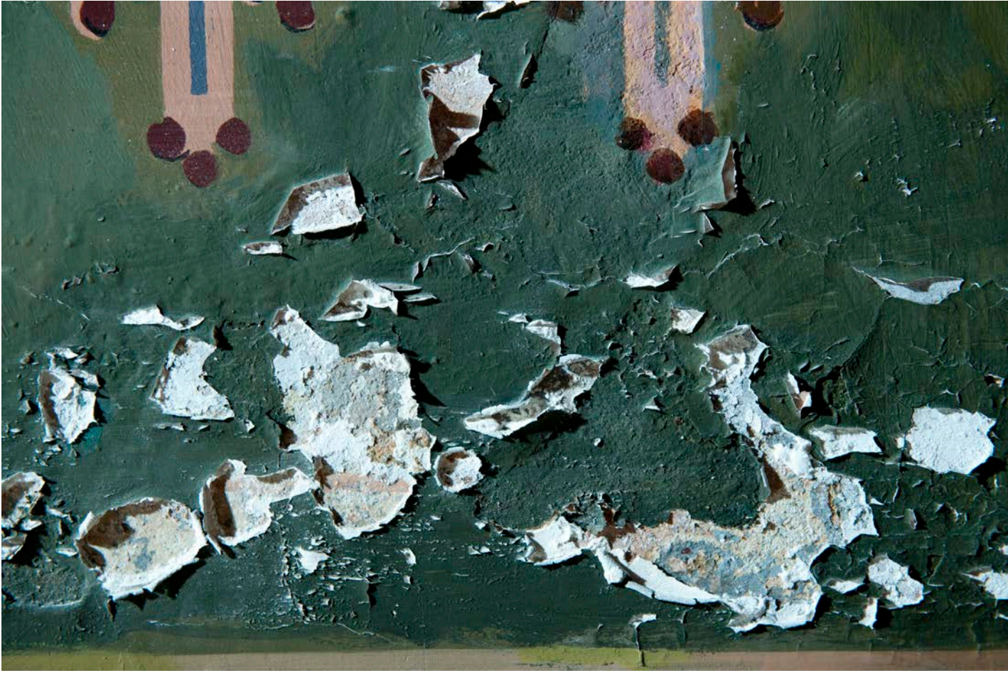
Partial detachment of paint layers, Marin Držić Theatre, Dubrovnik (Croatia) 20th century; Photo: 2011, HRZ (Katarina Gavrilica)
