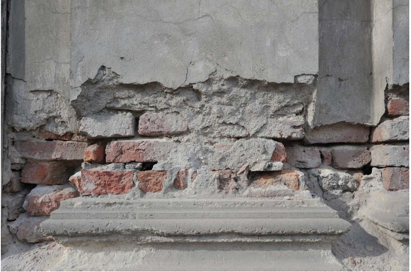
Crumbling building façade, Cluj-Napoca (Romania), 19th century; Photo: 2015, UAD (Adrian Rauca)
