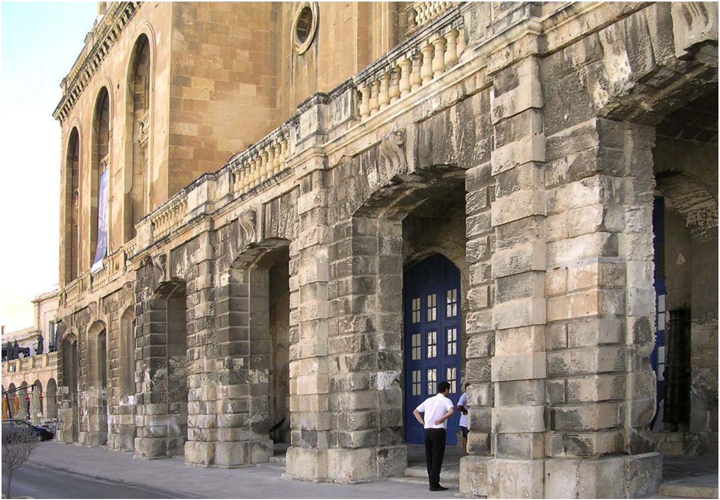
Blackened building due to air pollution (main façade, lower storey in Coralline Limestone), Maritime Museum (Old Naval Bakery), Birgu (Malta), 1842-1845; Photo: 2008, UM (JoAnn Cassar)
