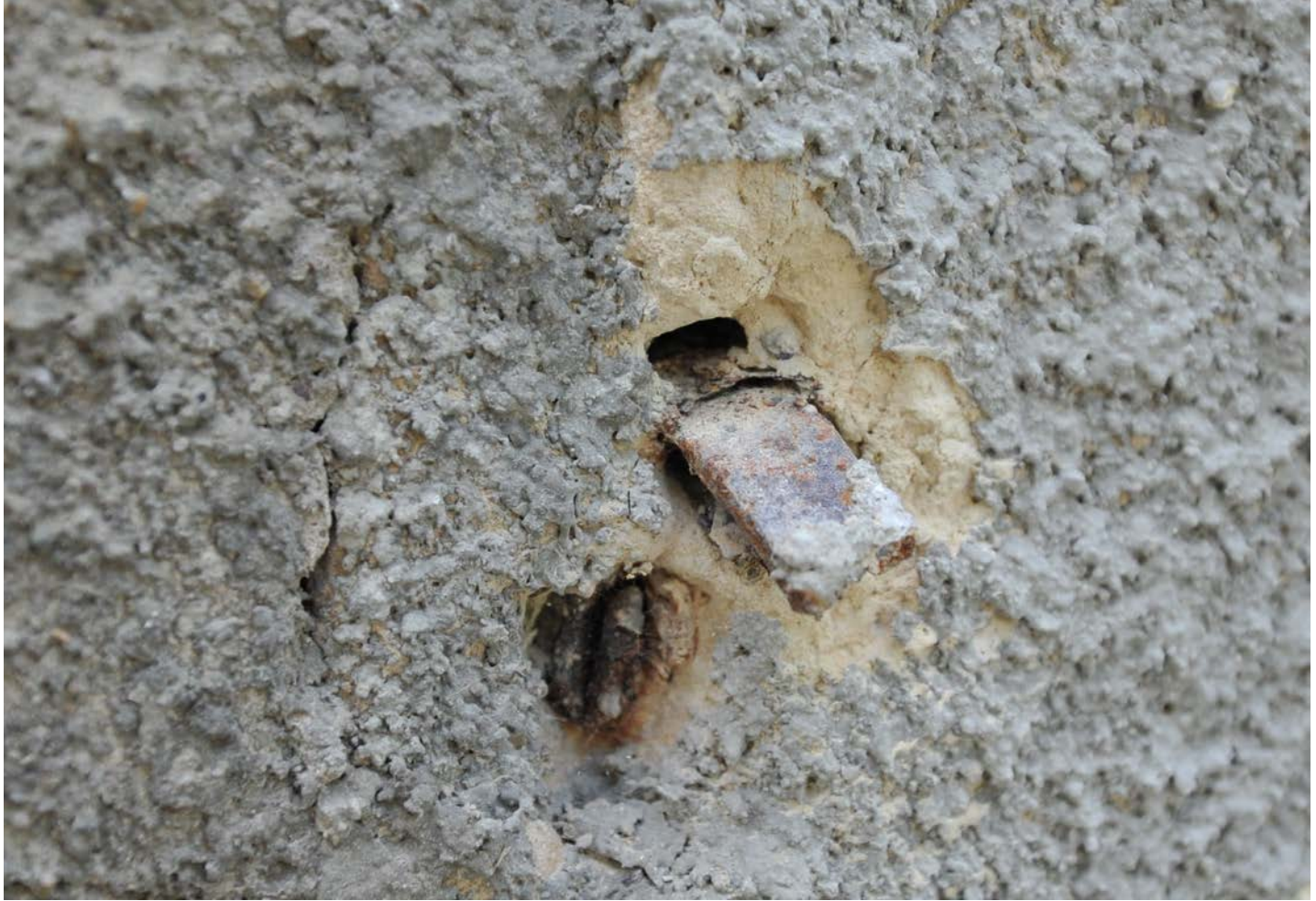
Corroded metal, building façade, Cluj-Napoca (Romania), 20th century; Photo: 2015, UAD (Adrian Rauca)
