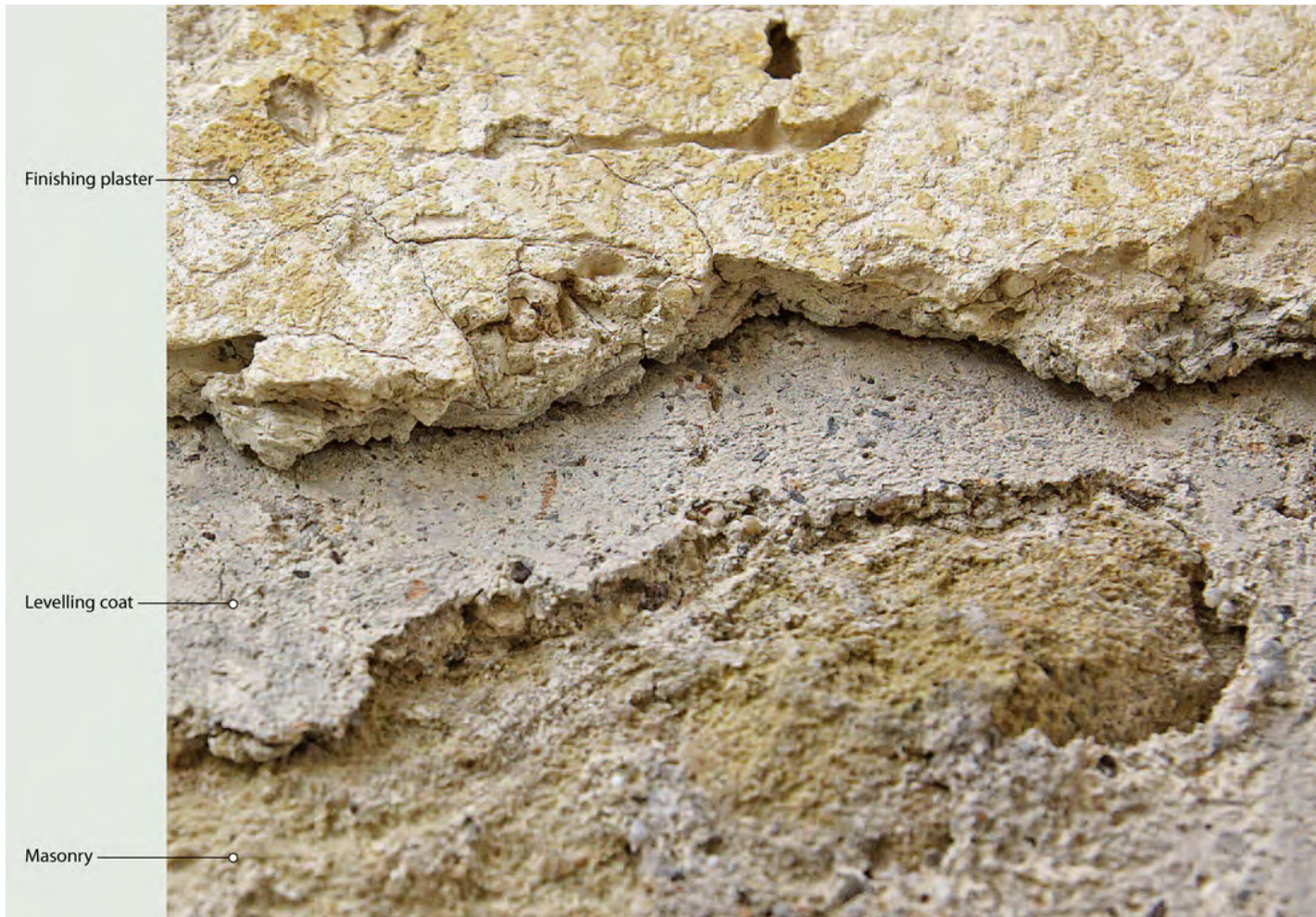
Levelling coat between masonry and finishing plaster (detail), Church of St. John Aliturgetos, Nessebar (Bulgaria), 13/14th century; Photo: 2014 (Stefan Belishki)
