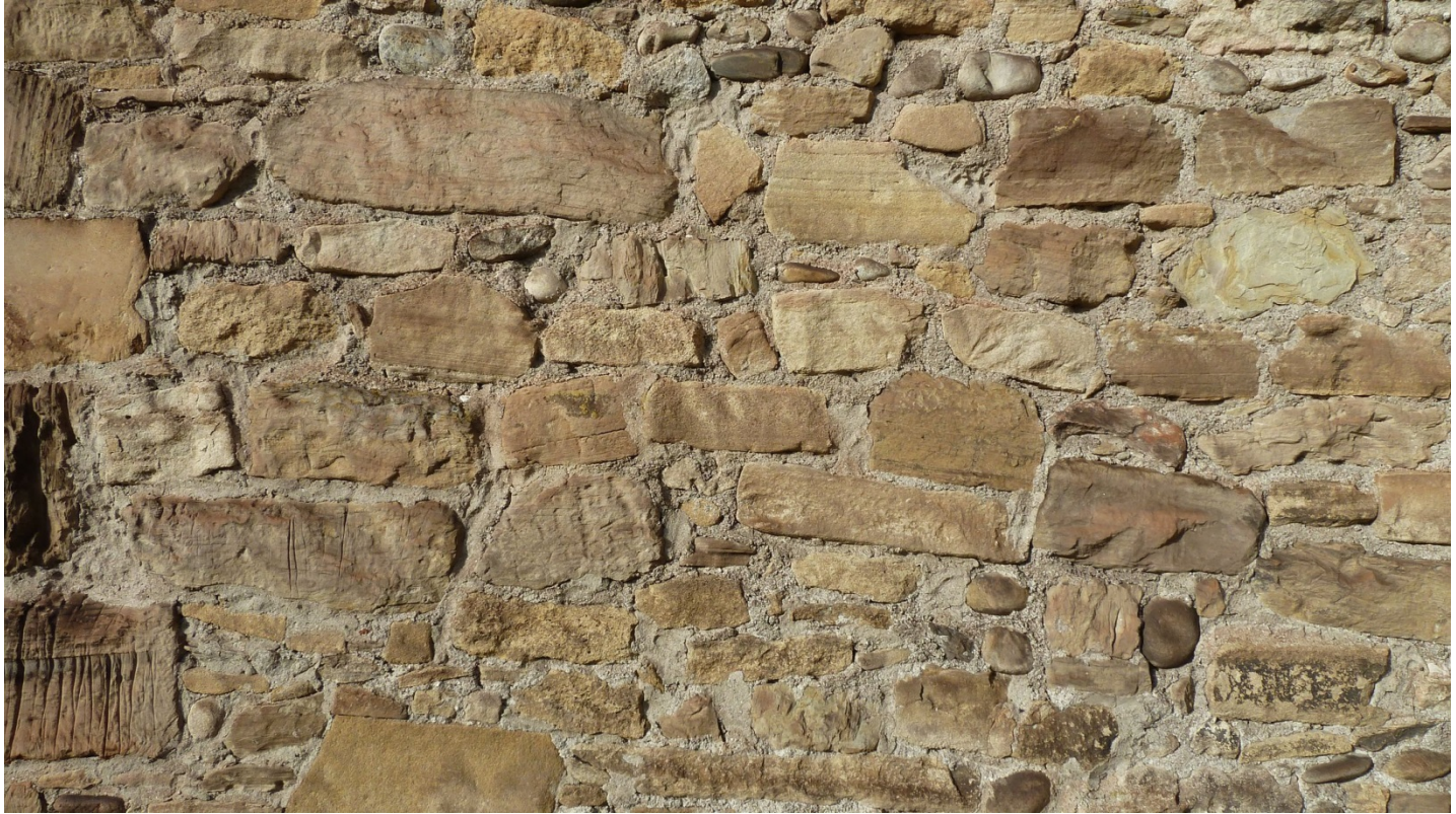
Mixed stone construction, southern façade, Dormition of the Theotokos Church, Strei (Romania), 13th century; Photo: 2015, UAD (Adrian Rauca)
