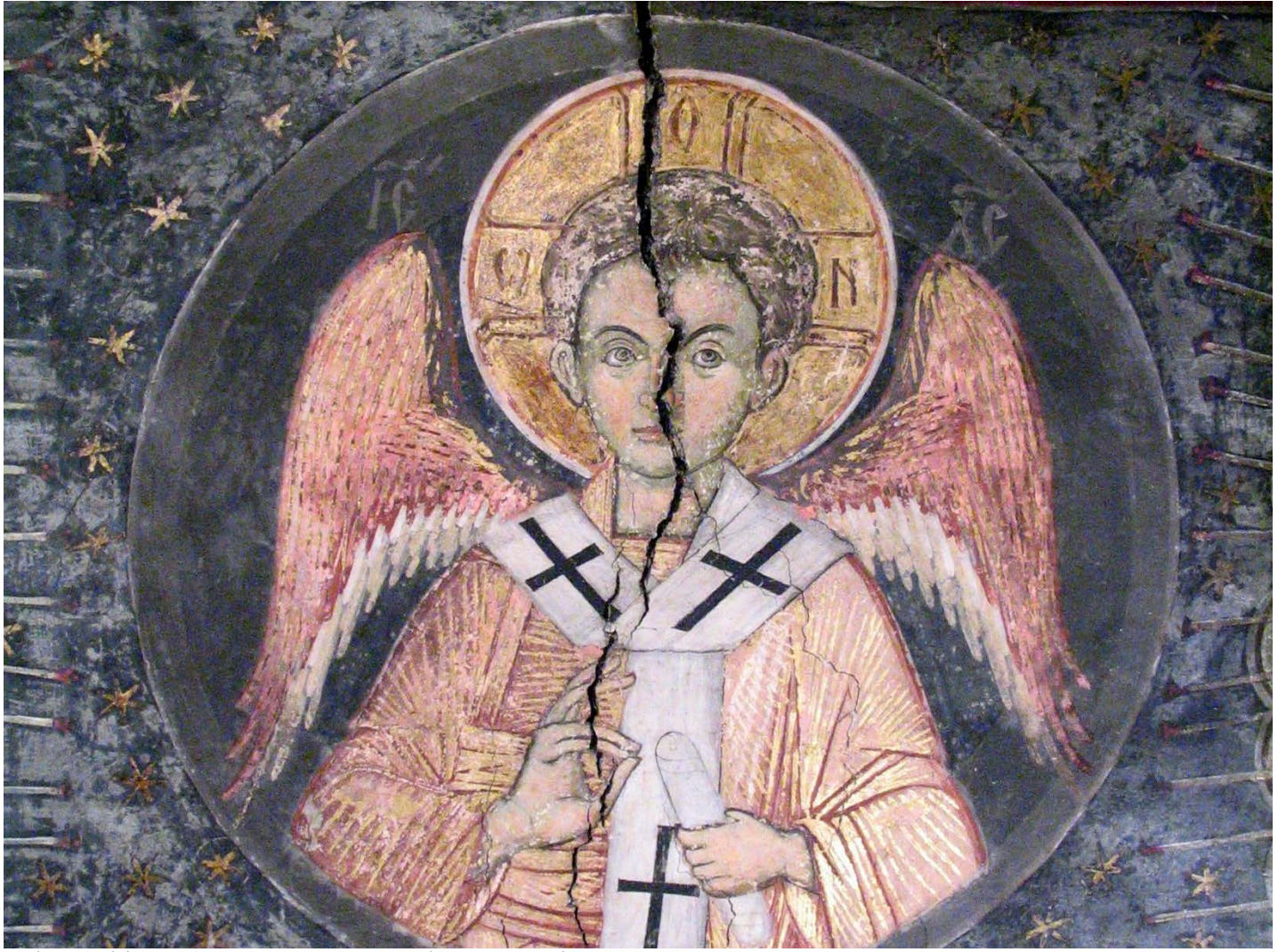
Crack in painted plaster, Sucevița Monastery (Romania), 1585; Photo: 2003, UAD (Adrian Rauca)
